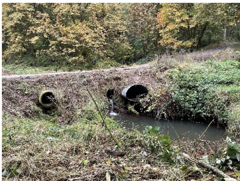
Before: Perched culvert restricting fish passage Photo credit: ODF
